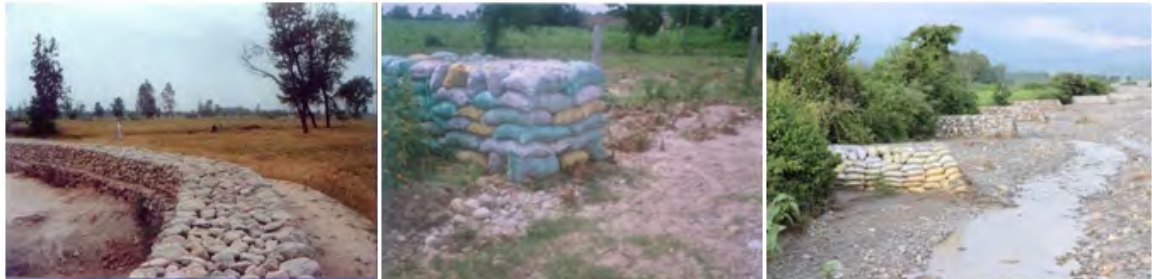
Gabion protection wall, Katta crate and spur structures for torrent control at Sabhawala village
